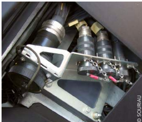
Closed electrical areas
